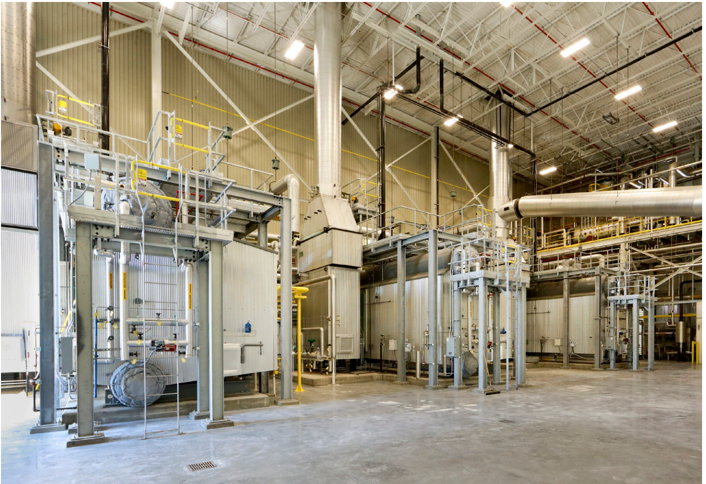
New dual-fuel boilers enhance steam system efficiency.
