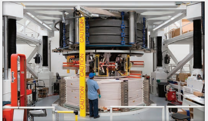
At this stage of turn insulation, half of the module is suspended, and half is already wrapped with insulation tape. Image credit: General Atomics
